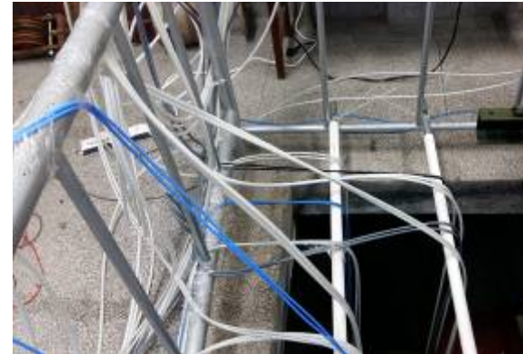
cables on the ground
