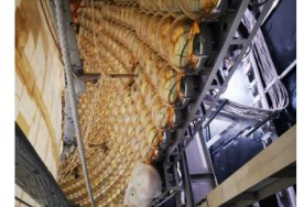
Installed PMT modules
